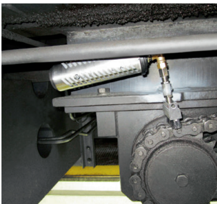
The 250 ml simalube lubricator lubricates the chain drive of a railway crane. The dispenser is also protected by a protective cover.
