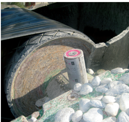
Belt drive lubricated with simalube.
