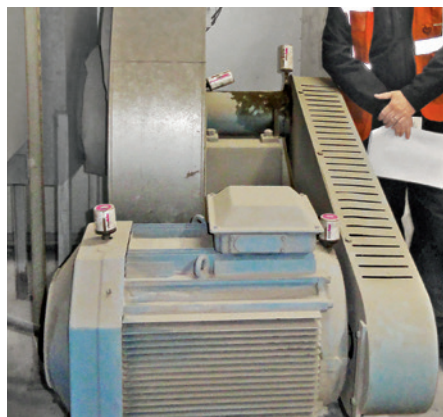
A combustion fan lubricated with two 60 ml and two 125 ml simalube lubricators.
