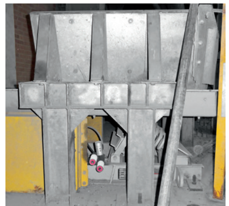
A vibrating conveyor lubricated by several 125 ml simalube lubricators.
