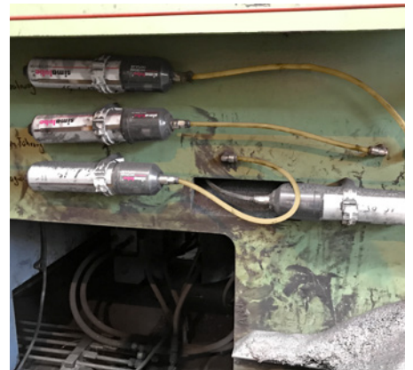
Thanks to the simalube IMPULSE pressure booster, the lubrication points at the winder (bearings, guide bushes and interlocks) can be installed remotely and supplied with lubricant via a hose installation.
