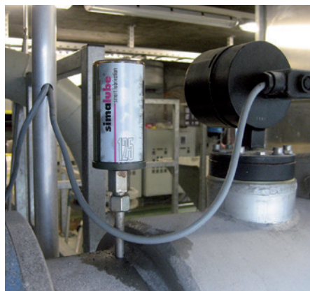
Lubricating bearings: the lubricant is transported to the bearings via a short pipe.
