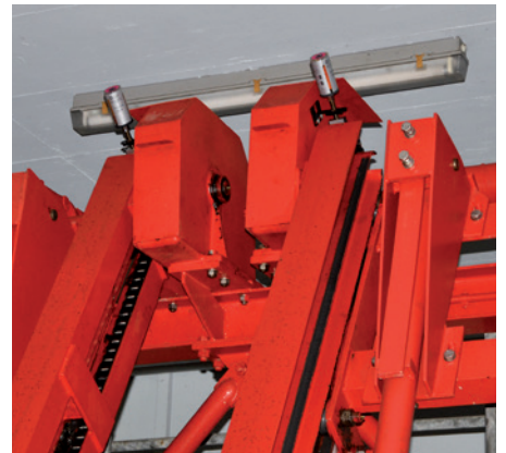
Chain lubrication with simalube on a bar screen equipped with brushes.
