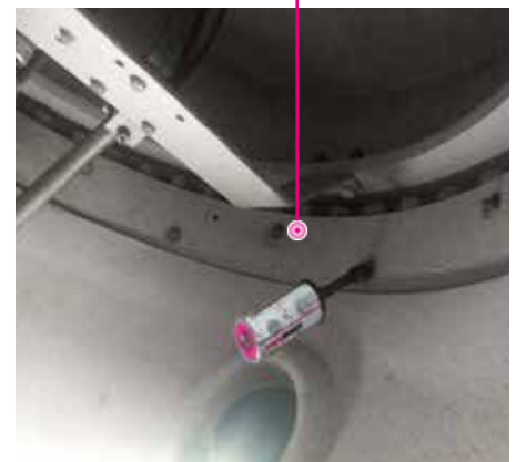
Automatic lubrication using the simalube 125 ml on a rotor blade bearing.
