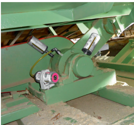
The bearings of a vibration channel are lubricated continuously by three lubricators.
