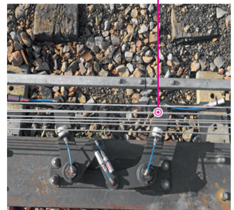
Two 30ml simalube lubricators and four 15ml simalube dispensers continuously lubricate the compensator of a signalling system.
