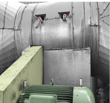
Lubrication of the bearings of a ventilation unit with 125 ml and 15 ml simalube units.
