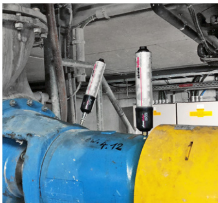
The bearings of the pump are lubricated with two IMPULSE and 250ml simalube units.
