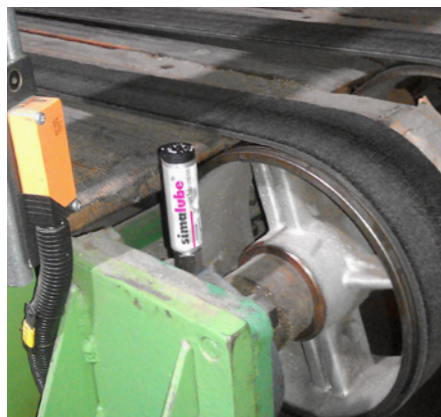
The bearings of the transport belts in a corrugated cardboard factory are continuously lubricated with the simalube lubricator.
